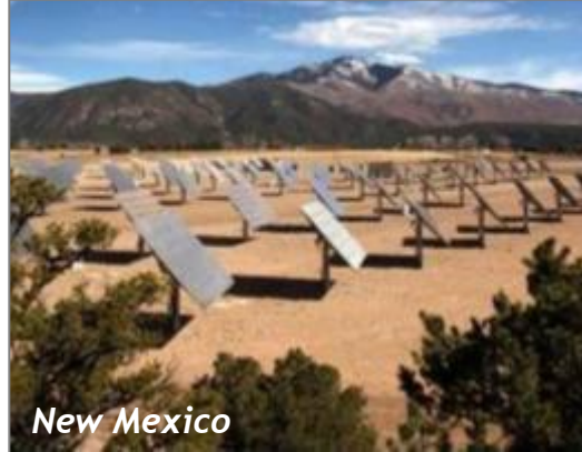
Concentrators installed on remediated mine tailings
