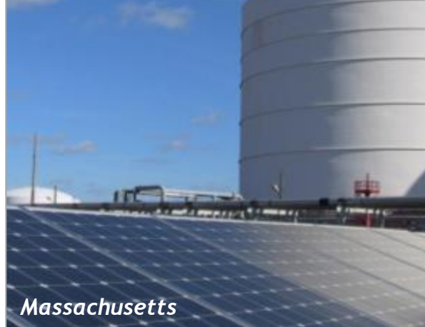
Solar array at former manufactured gas plant
